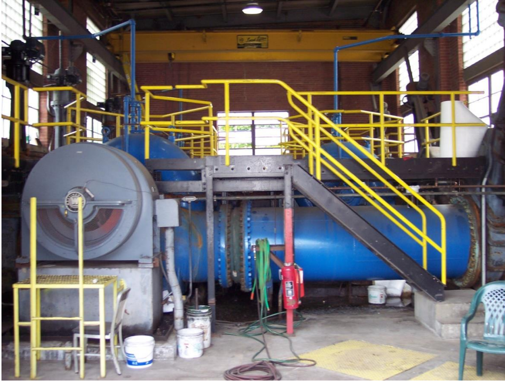
Figure 2-3 Greenidge Unit 4 circulating water pump A. Pumps B and C are behind Pump A.
