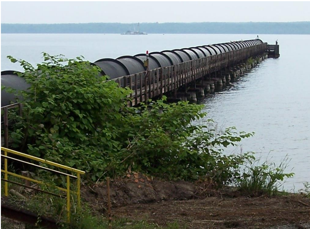
Figure 2-2 Greenidge Unit 4 intake pipe
