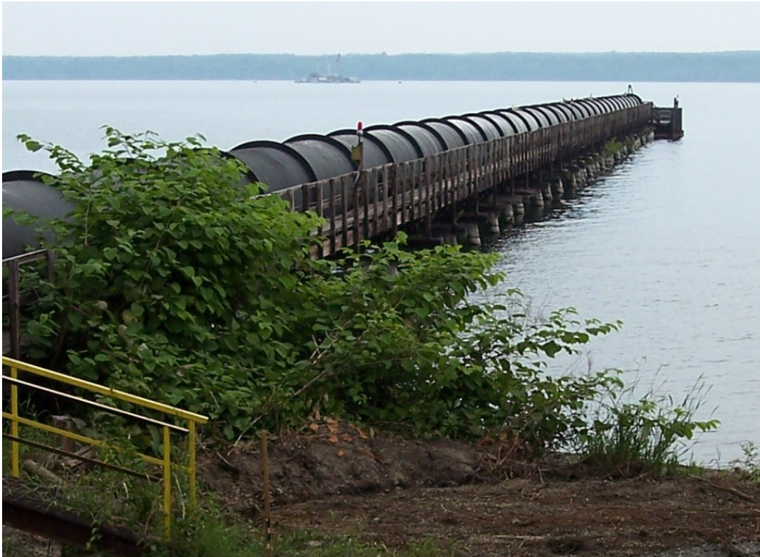
Figure 2-1 Unit 4 withdraws water from an elevated 7-ft diameter conduit that extends 650 from the west shore of Seneca Lake.
