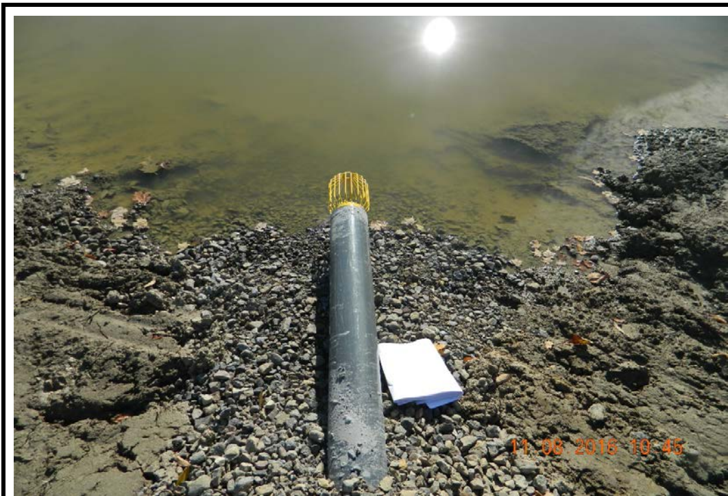
Photo 39: Riser Structure orifice pipe and Agri Drain Bar Guard, looking east (11/8/16)
