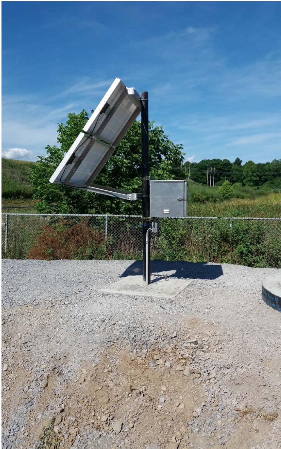
Photo 17: Solar Power System and Battery Box (6/30/16)
