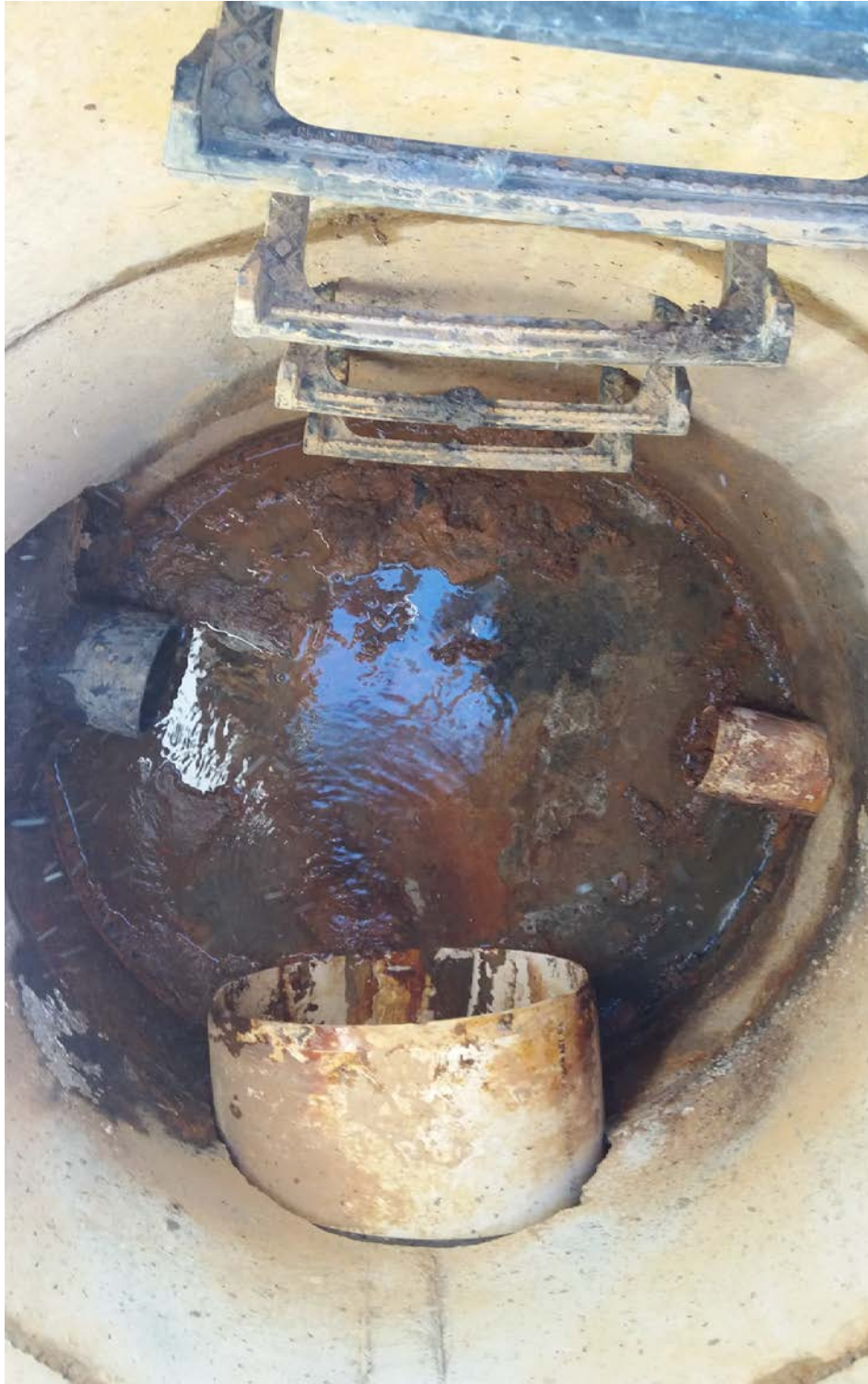
Photo 8 - Modified MH I/II/S-1 (6/30/16)
