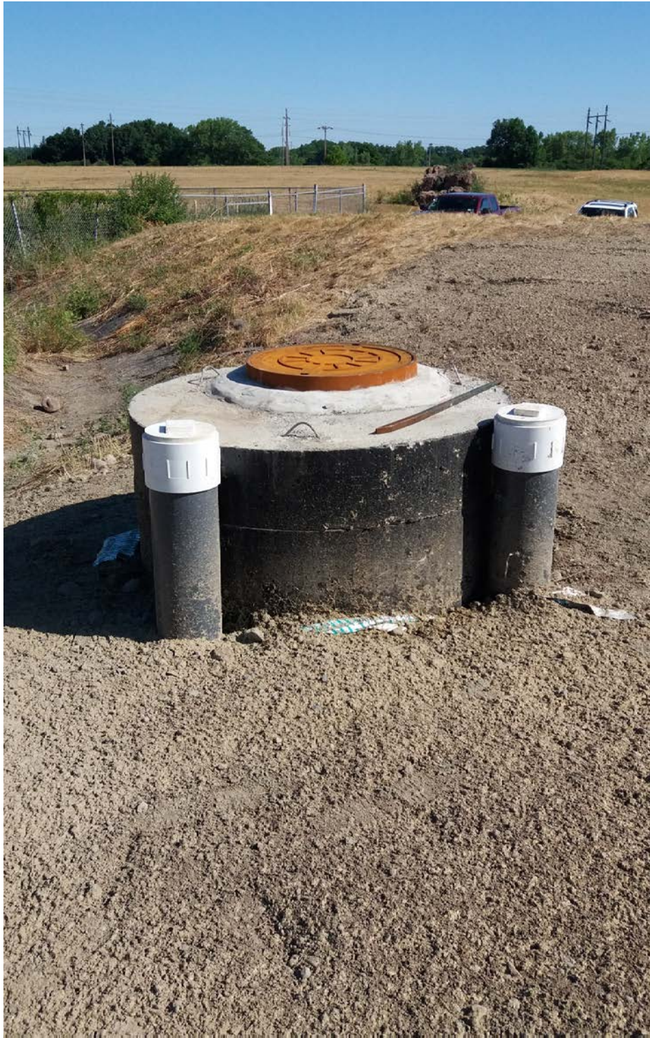
Photo 6 - MH COMMON-1 and eight-inch cleanouts (6/30/16)
