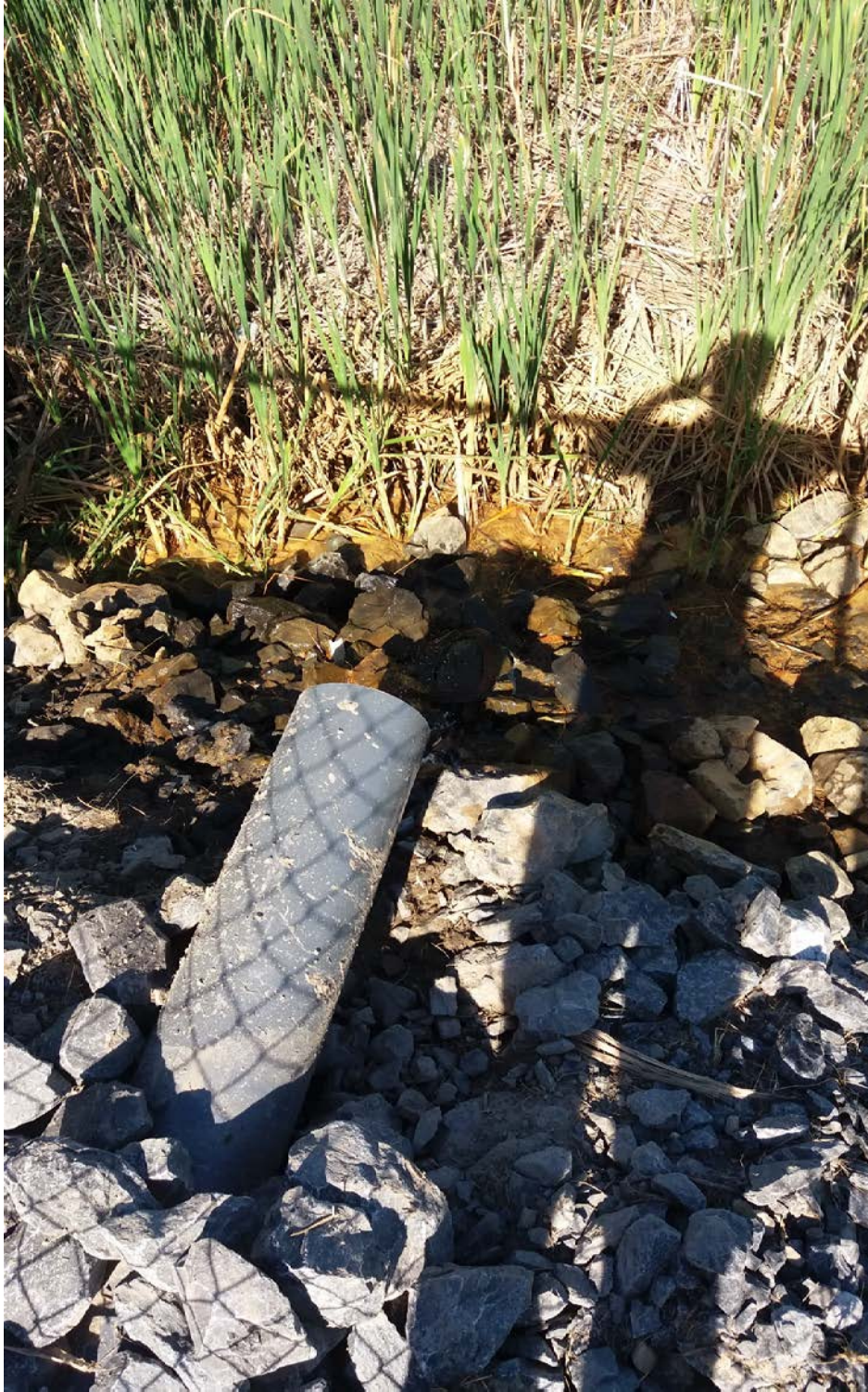
Photo 14 - Eight-inch discharge to Leachate Pond (6/30/16)
