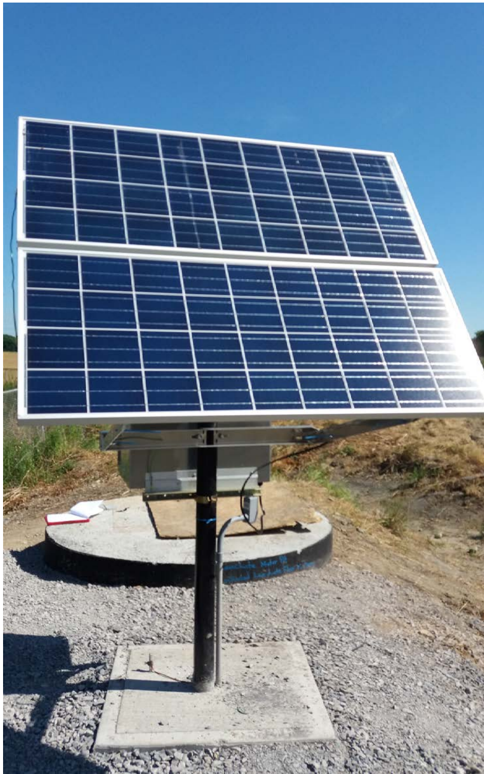
Photo 18 - Solar panels and Leachate Meter Pit (6/30/16)
