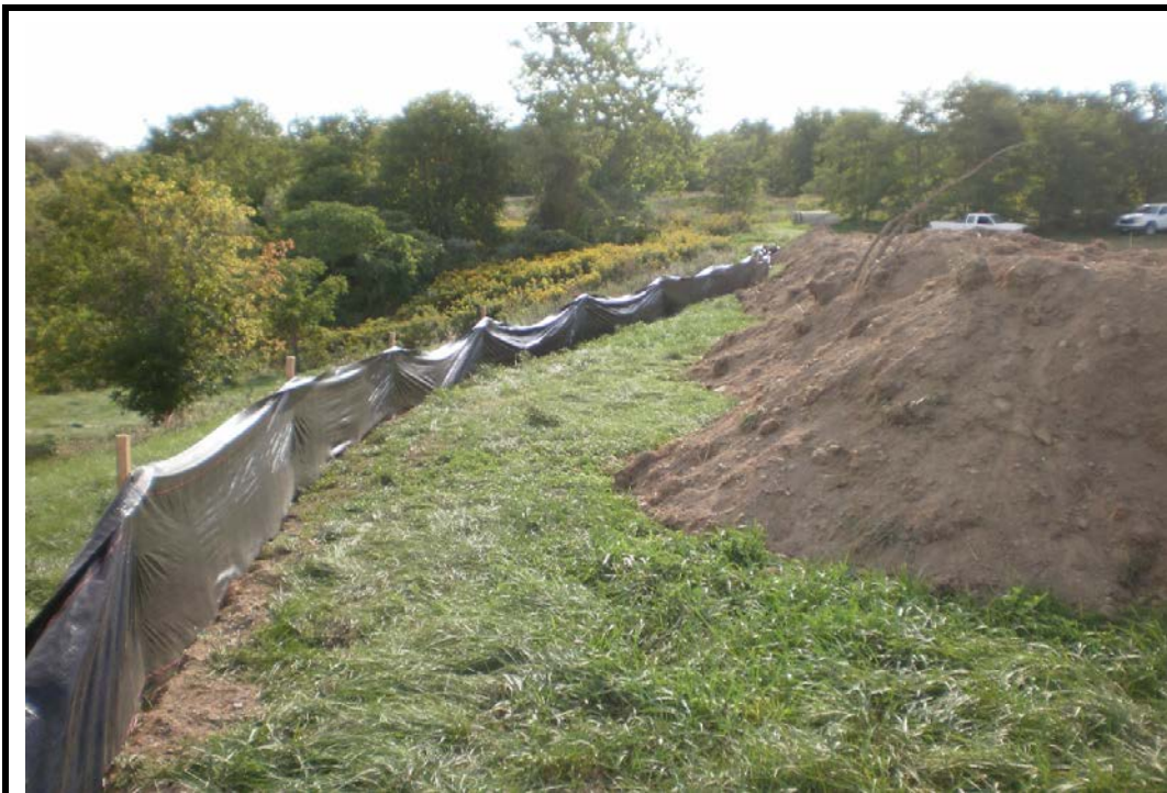
Photo 25: Silt fence installed east of Leachate Pond, looking east (9/26/16)
